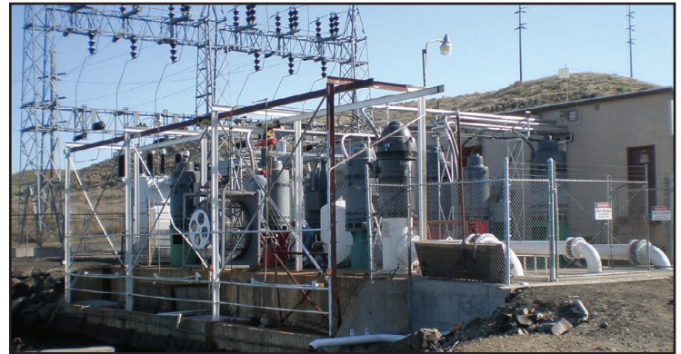
NPC Pump Station located at the potato farm.
